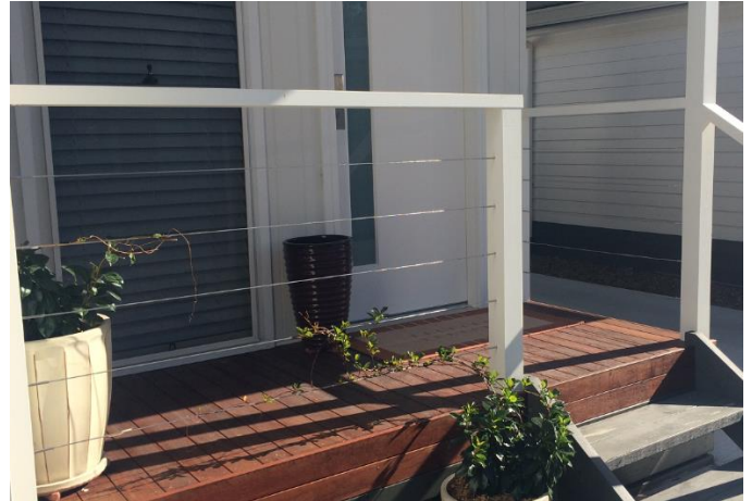
(Handrails not painted)
